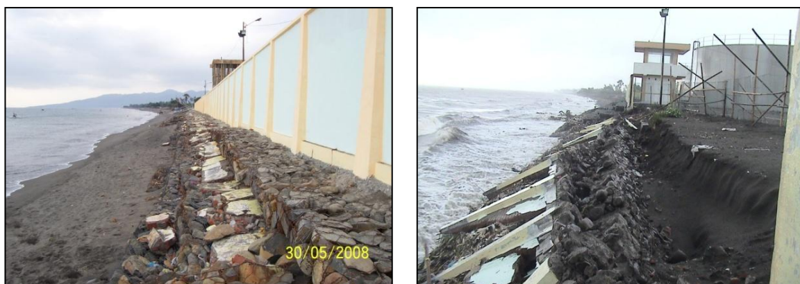
Figure 2. The beach erosion on the west boundary wall of ADPP.
